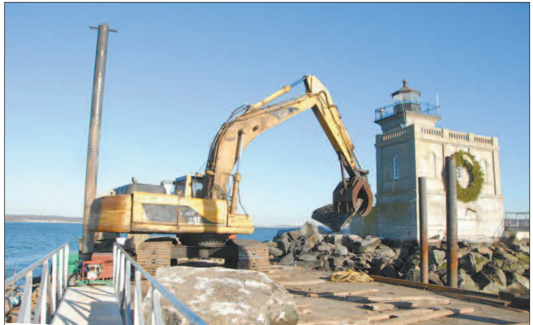
Repairs to Huntington Lighthouse may have to wait until the fall, depending on the findings of a preconstruction exploration work crew, pictured Friday.
